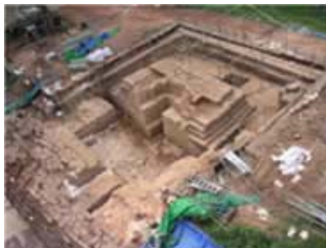
北側の基礎部にトレンチを入れ調査 Research by setting a trench ※2 in the foundation of northern side
